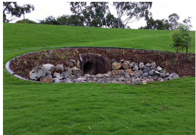
Figure 33: Secondary drainage pipes
