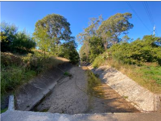
Photograph 21: The concrete canal which follows the original creekline. View to east from Russel Street.
