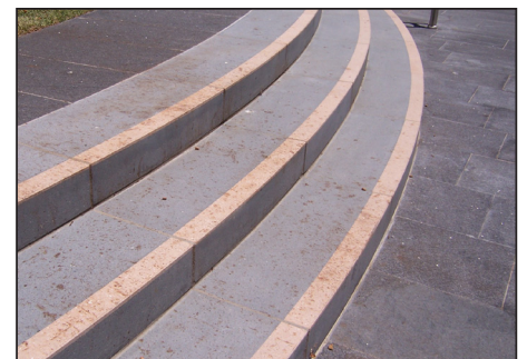
Change of level well integrated into public domain - precast steps, Memory Park, Penrith
