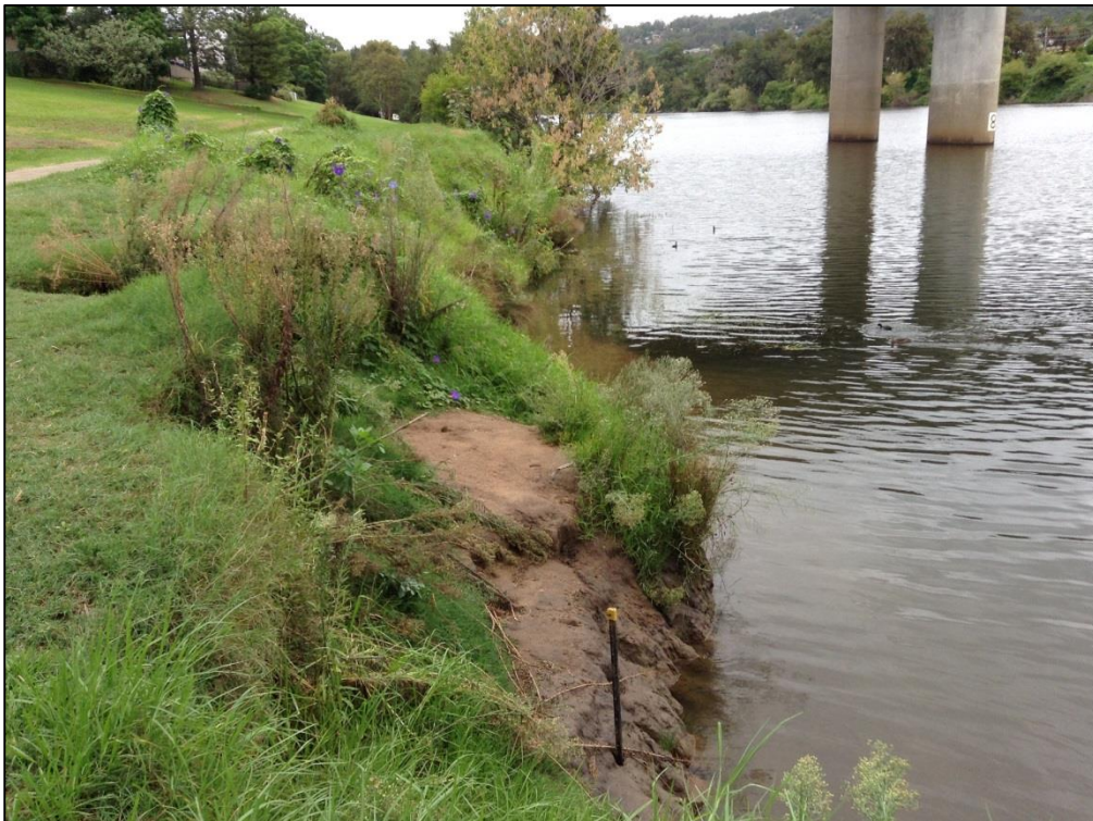
Plate 1: Bank erosion, weeds and poor habitat provide opportunities for improvement
