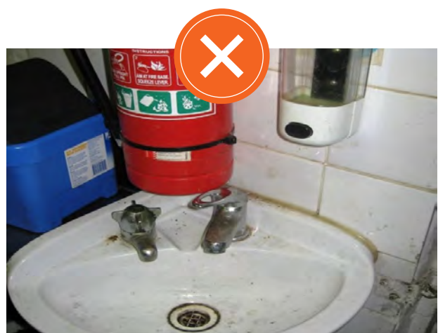
No soap or single use towels provided hand basin. Penalty Notice issued.
